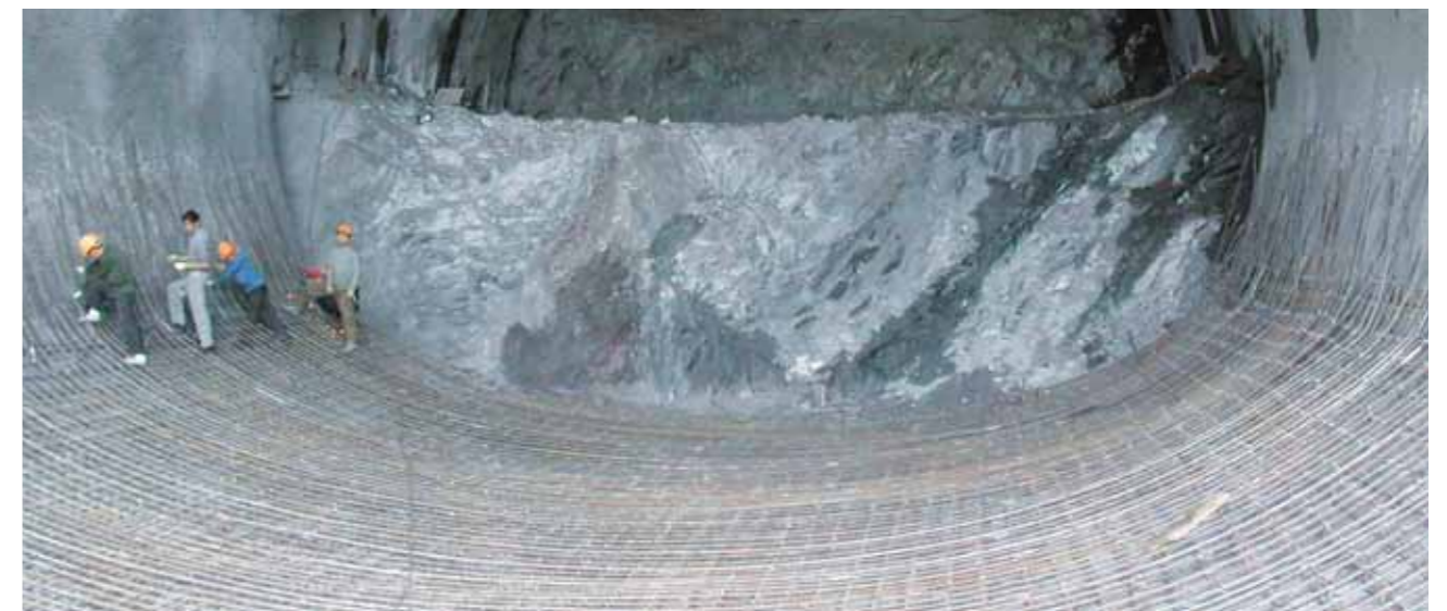
14 Two-bench mining in Devonian quartzites with invert reinforcement near the north entrance
